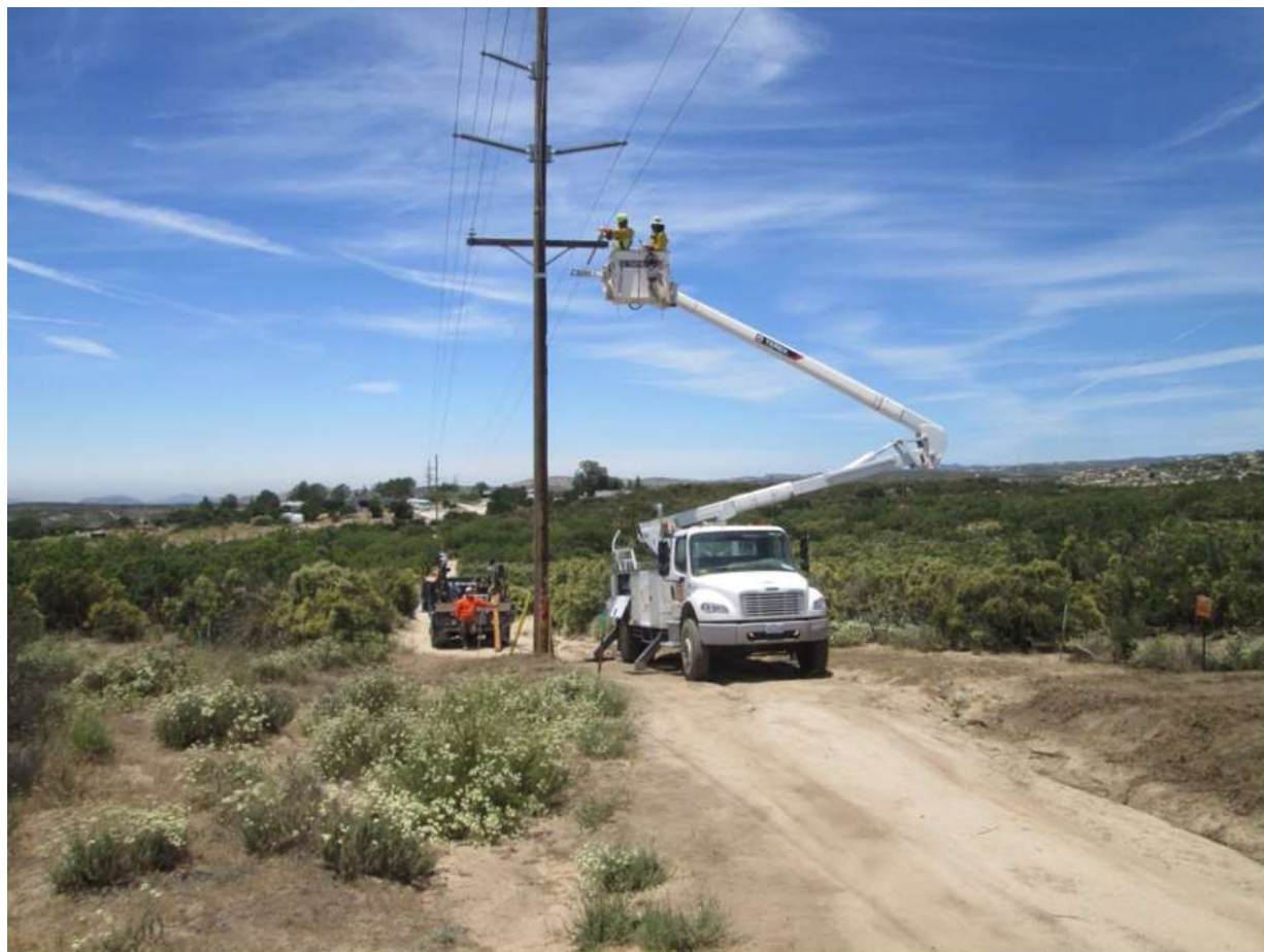
Photo 5: Construction crew observed spreading wire at Z44267 (TL 6931) to allow the overhead space necessary for pole hole drilling. Crews were observed staying within existing access roads and delineated work spaces (MM BIO-1).
