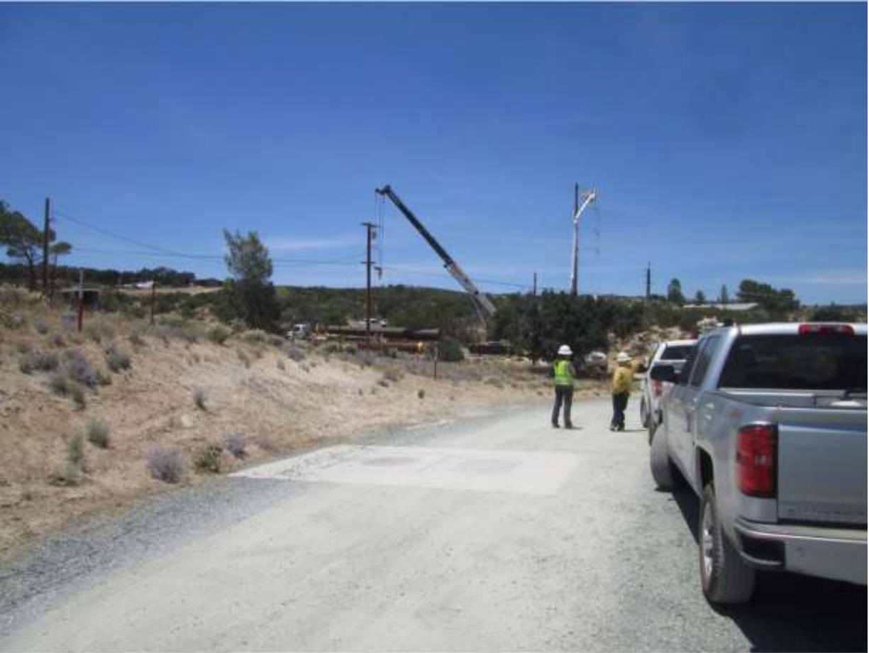
Photo 4: During installation of grounding and staging of a steel replacement pole at Z44294 (TL 6931), a biological monitor was observed spot checking the activity in accordance with MM BIO-3 and MM BIO-22, and a fire patrol was observed inspecting the site for compliance with the CFPPP (MM FF-1).
