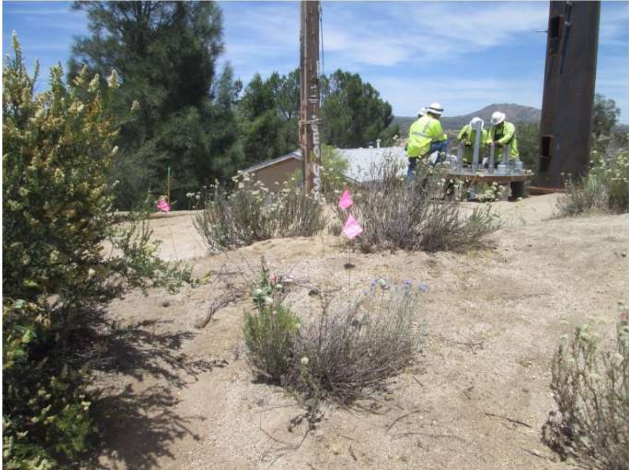
Photo 2: During foundation setting at Z44293 (TL 6931), designated plants were flagged for avoidance in accordance with MM BIO-13 and MM BIO-14.
