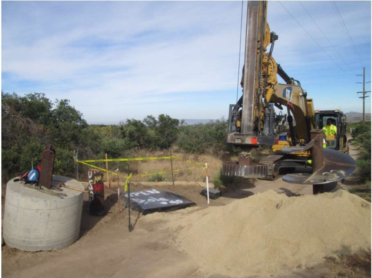
Photo 3: After completion of conventional drilling for pole P46409 (TL 6931), the hole was securely covered for safety and to prevent wildlife entrapment in accordance with MM BIO-23.
