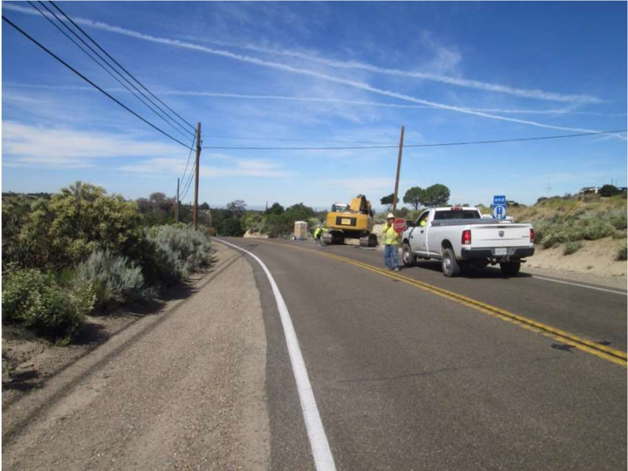
Photo 6: During the transport of a drill from Z44266 to Z44263 (TL 6931), traffic control flag persons were utilized to direct traffic around the equipment while traveling along a section of Highway 94 in accordance with APM TRANS-02.
